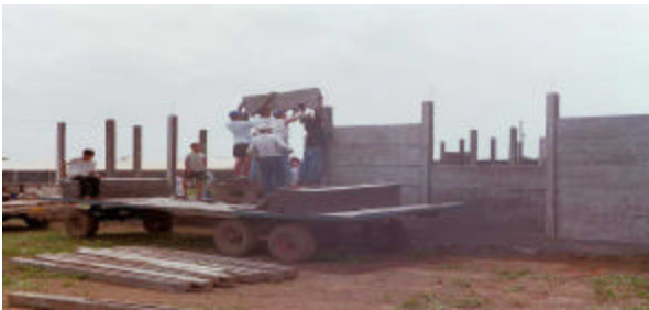
Ms. Kruse (standing back left) helping to hoist a concrete block into place...future health clinic in Nueva Vida
