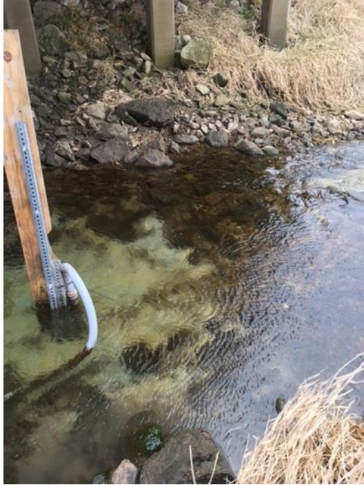
Figure 64. Streambed scouring and bare clay beneath the pressure transducer at Site 5 after Storm 17. Note the transition from the scoured pool section of the stream to the run with larger cobbles and boulders.
