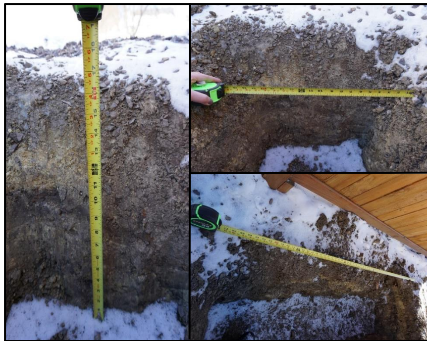
Figure 2. Measurements of depth, width, and length taken after completion of the trench.
