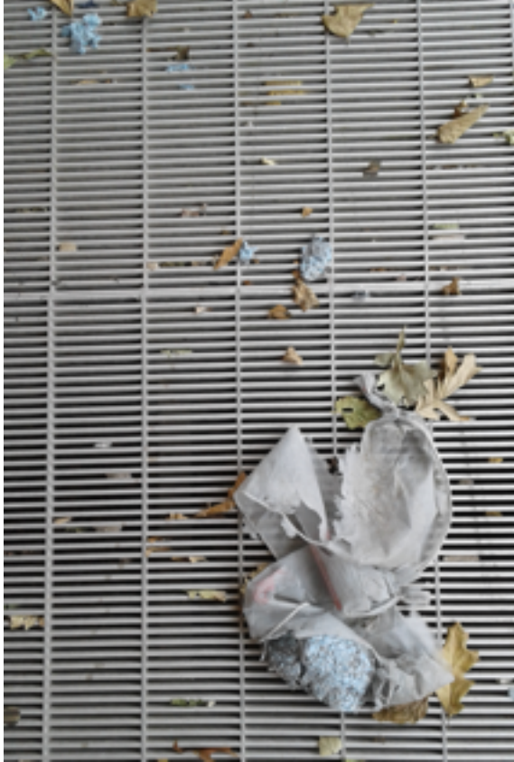
Figure A-11. Construction debris
